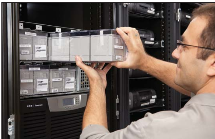
IT staff can easily replace battery modules.
