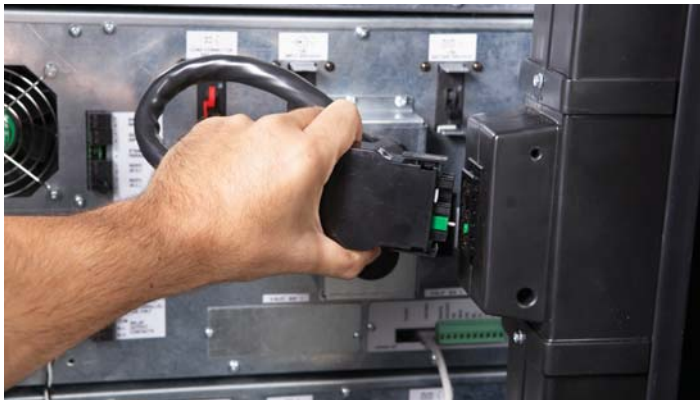
Adding modules is a simple plug-and-power procedure for IT personnel with safety-approved connectors.
