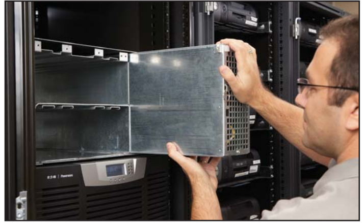
IT staff can easily install electronics modules.
