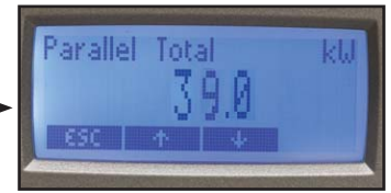
Display full system output from any UPS
